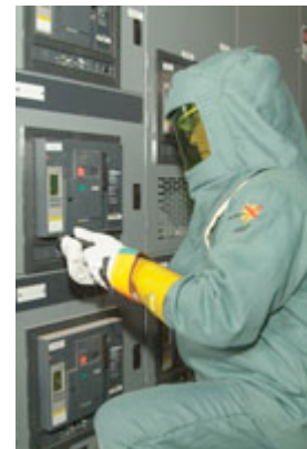
The minimum PPE requirements of NFPA 70E-2004 Hazard Risk Category 4 include protection such as an Arc40 coat, pants and hood with hard cap. The worker is preparing to rack a Square D Masterpact circuit breaker from its cell.
